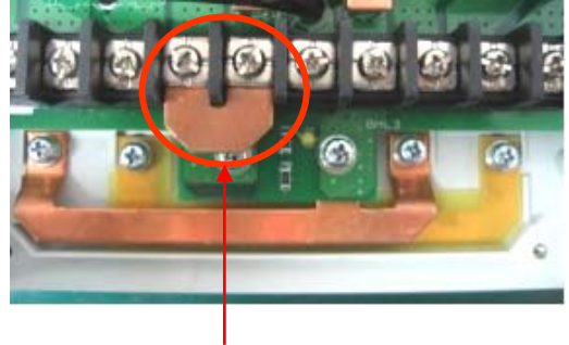
P1-B1 connection BUSBAR
