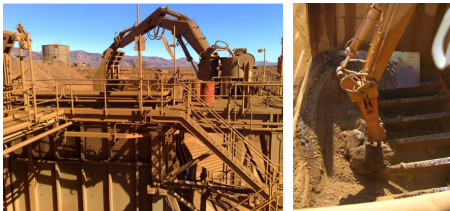
Fig. 1 Rock breaker (a) at rest over ROM bin (b) breaking a rock on grizzly.
